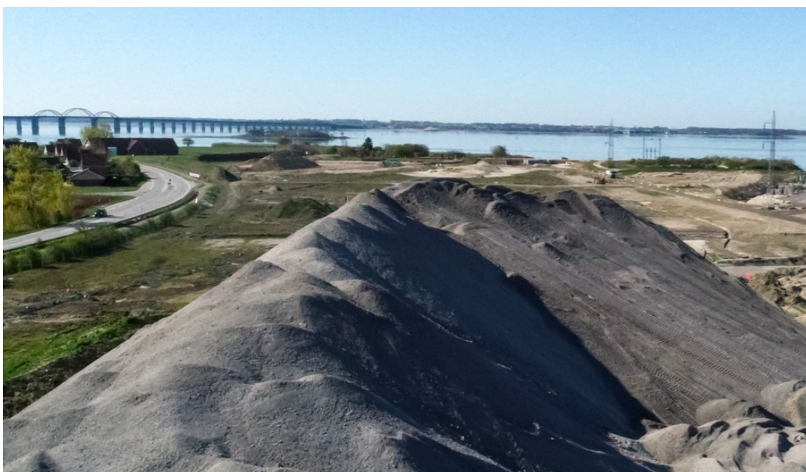
Construction site at Storstrømsbro with bottom ash gravel in stock ready for use in connecting roads to the new bridge.
